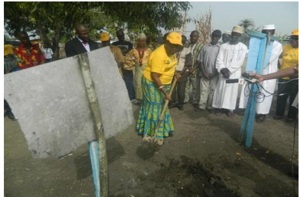
Figure 1 Justice Gladys K. Johnson breaking grounds for the construction of the memorial on Duport Road
